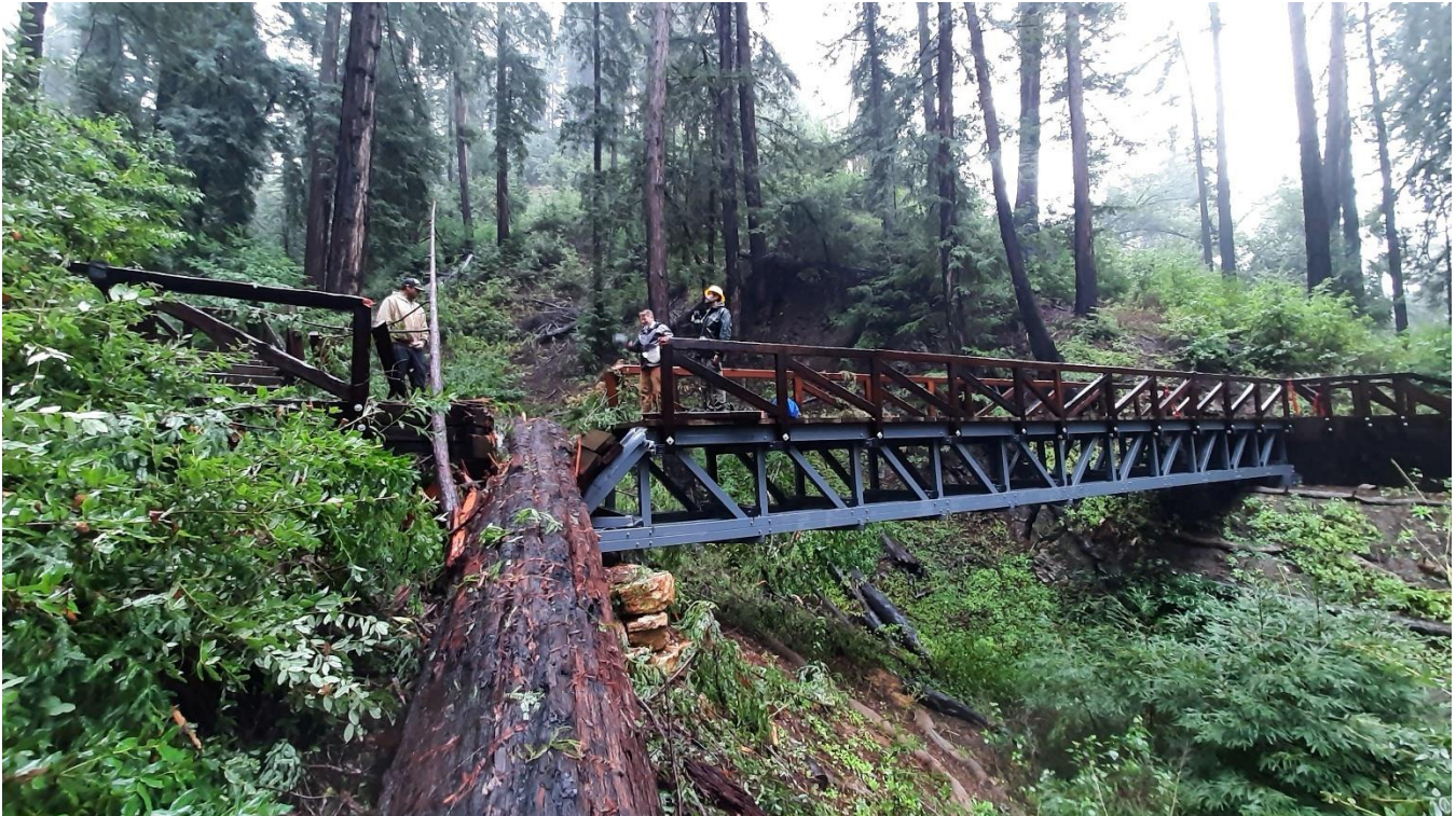
The Pfeiffer Falls Trail bridge was damaged by a fallen redwood tree in 2023, leading to a temporary trail closure. Photo from California State Parks
